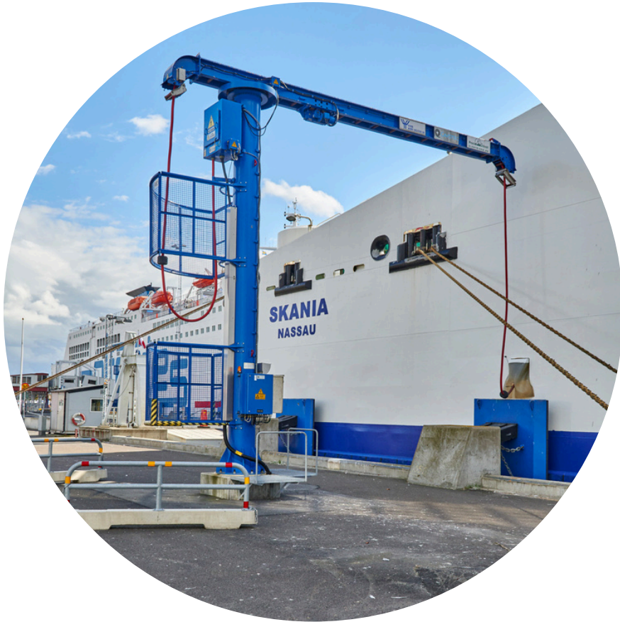
High Voltage Shore Connection 50 & 60 Hertz
